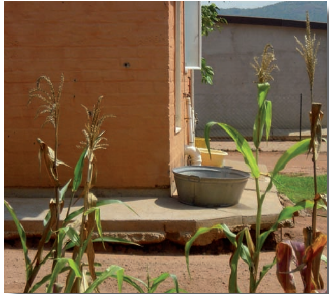
Soil erosion around house foundations in Sterkwater
