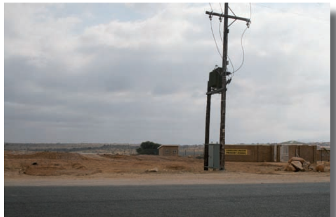
Open land next to the new school where the concrete batch was situated, July 2008
