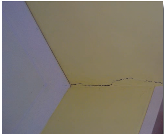
Cracks in a house in Sterkwater
